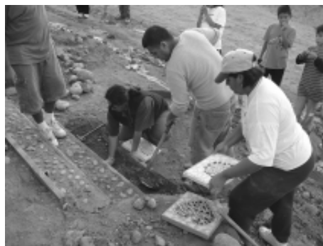
Students and Nuevo Milenio residents lay mosaic tiles at the site of an info-structure.
